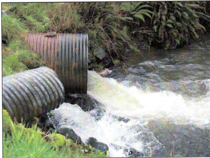
Figure 16 - Perched Culvert Example
