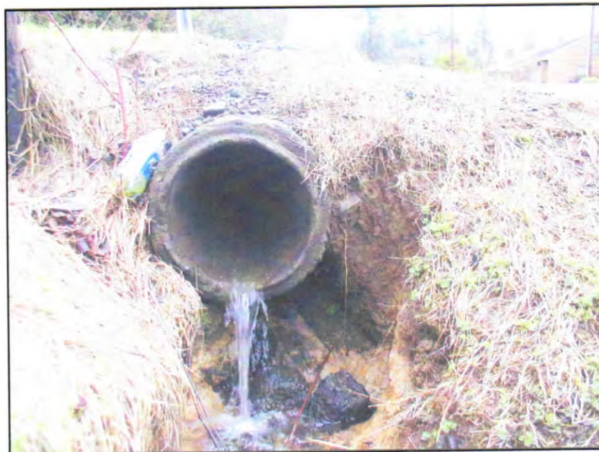
Figure 18 - Scoured Culvert Outlet
