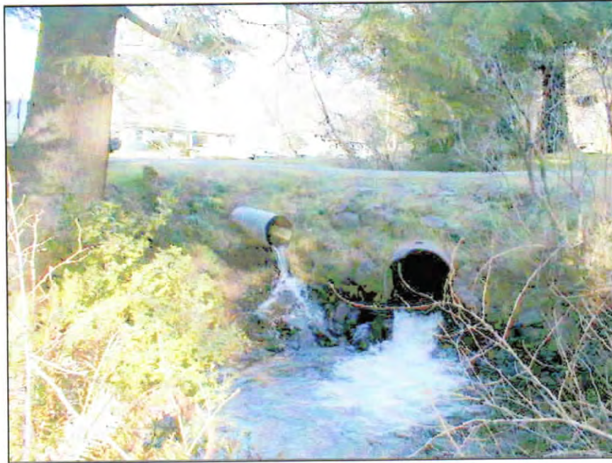
Figure 15 - Perched Culvert Example
