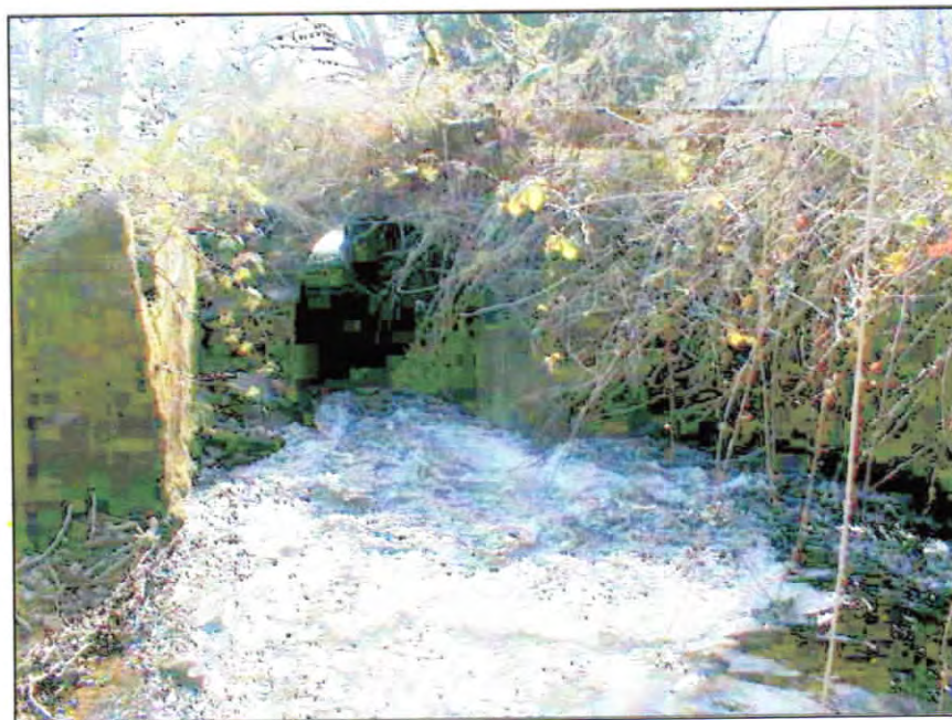
Figure 14 - Scoured Bottom Culvert
