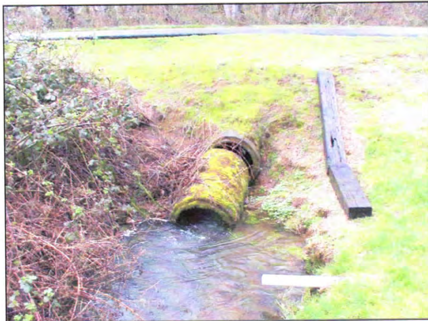
Figure 13 - Broken Pipes Example
