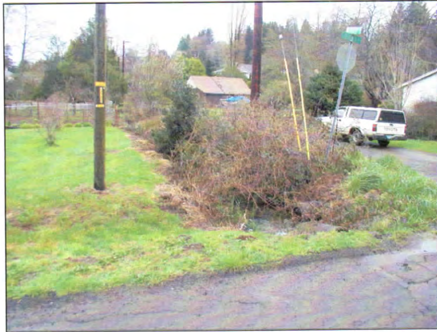
Figure 19 - Overgrown Ditch Example
