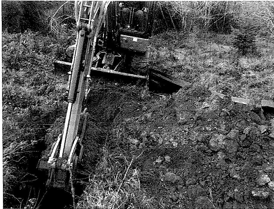
Photo 17 – View of the firm silty soils encountered during excavation of Test Pit-8.
