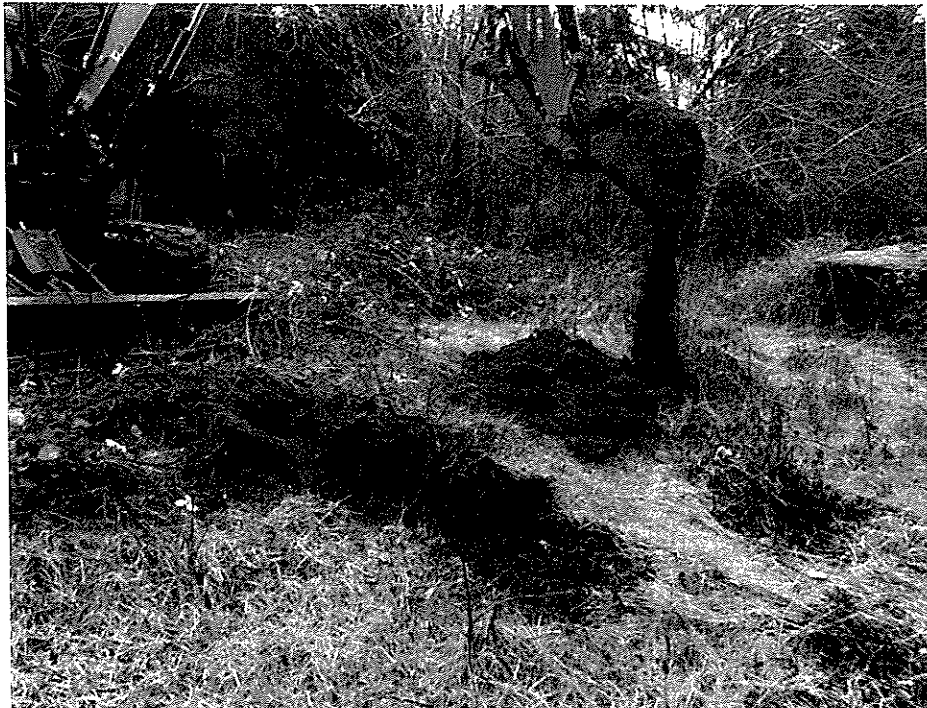
Photo 20 – View of Test Pit-12 during excavation in the area of the proposed pump station.
