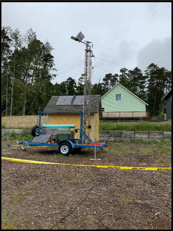
Temporary Antenna for communications
