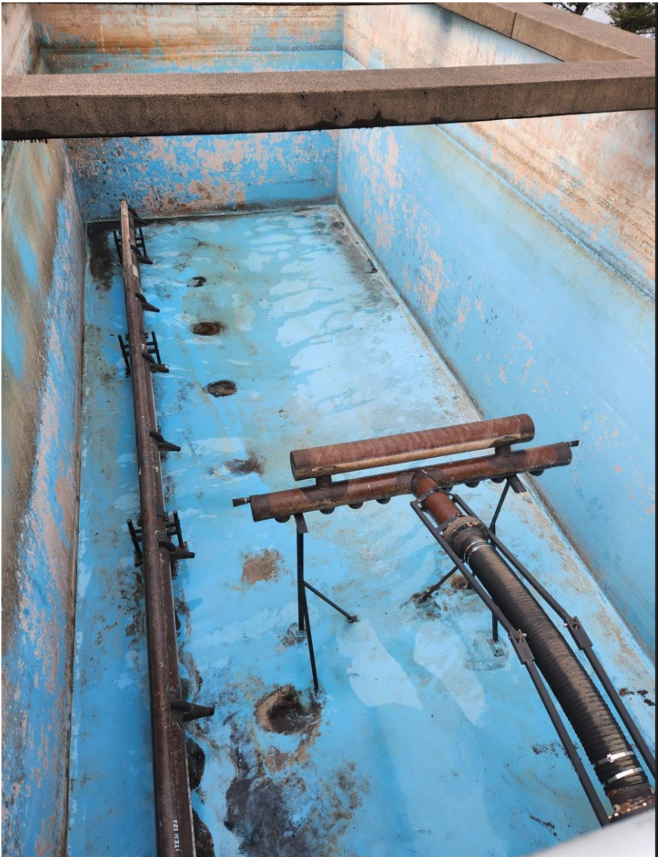
Sewer digester tank, emptied due to hole in pump base
