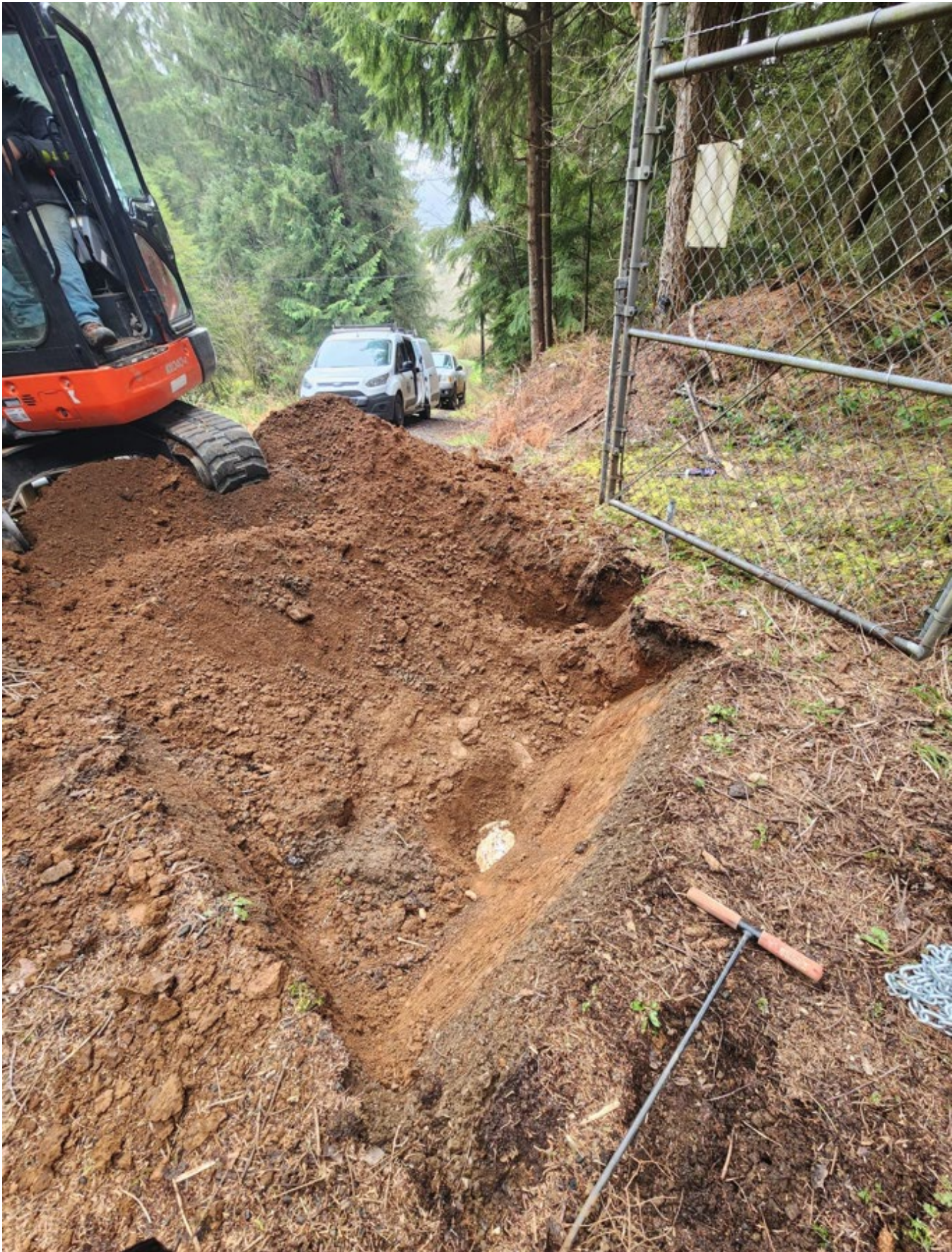
Finding the pipe location to know where to install the isolation valves on Juno Hill
