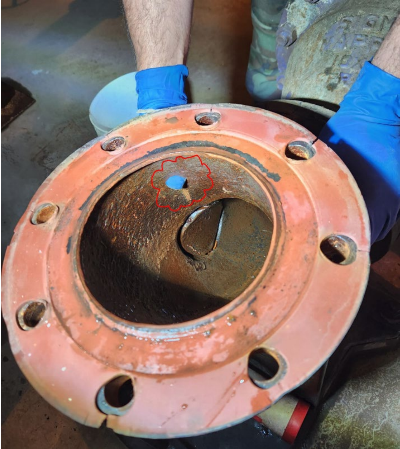
Hole worn thru pump base
