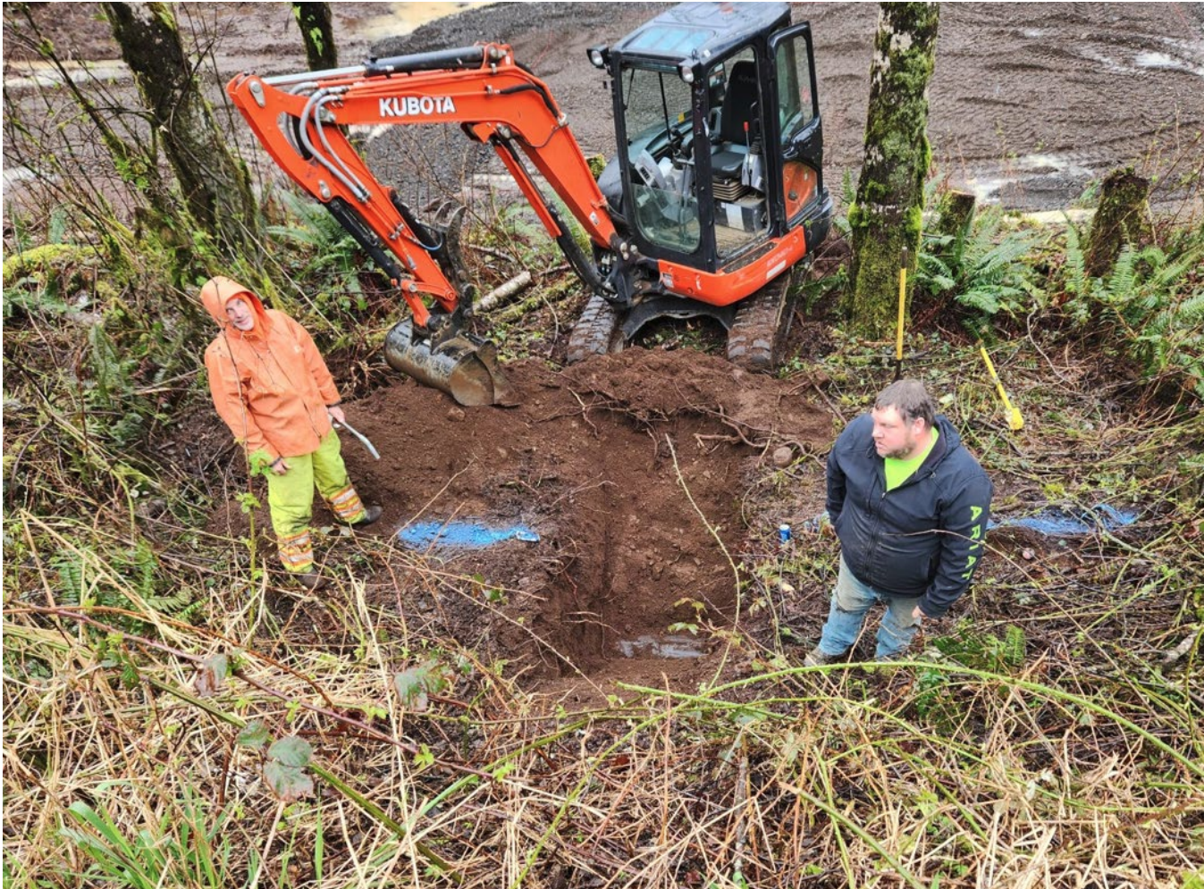
Found and exposed the 18 inch water transmission line along Kilchis River Logging Road.
