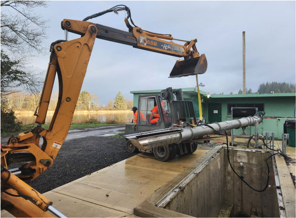
Removing screen from the vault to replace the brushes that become clogged
