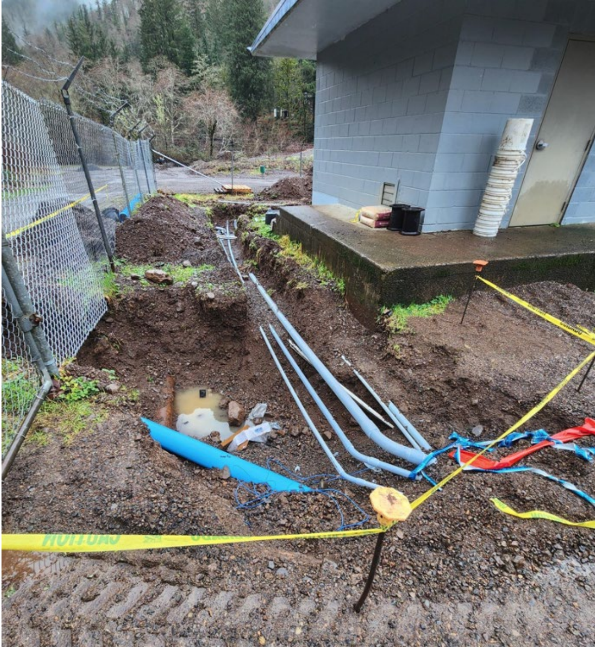
Electrical conduits at Well 3
