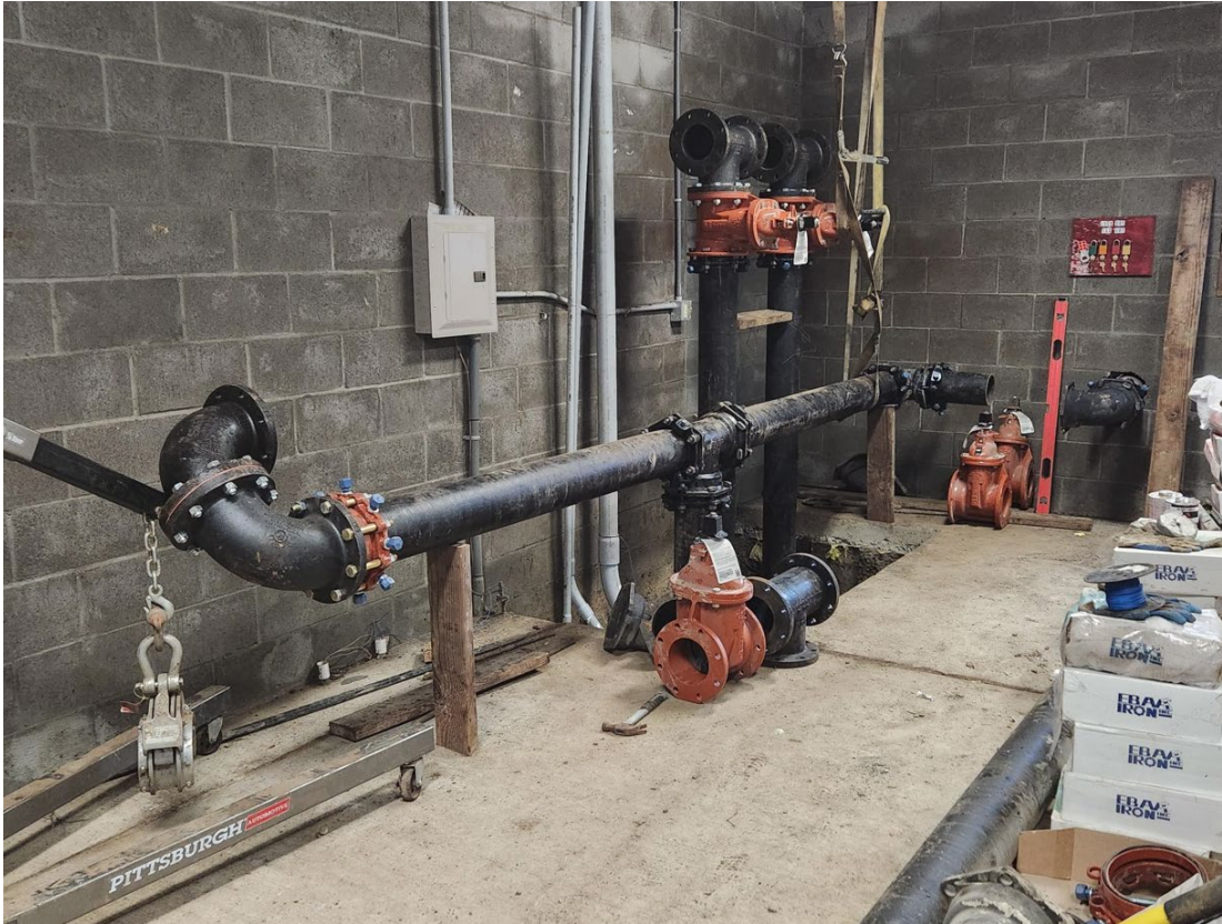
Piping inside the water building
