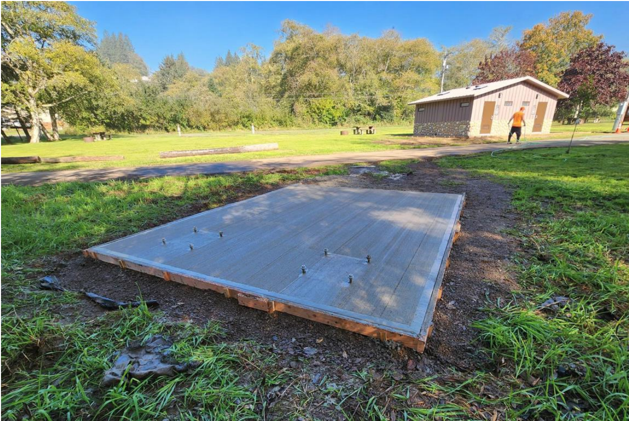
Placing anchor bolts in Bike Kiosk slab for lockers to fit upon
