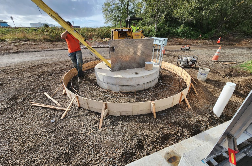
Sewer lift station
