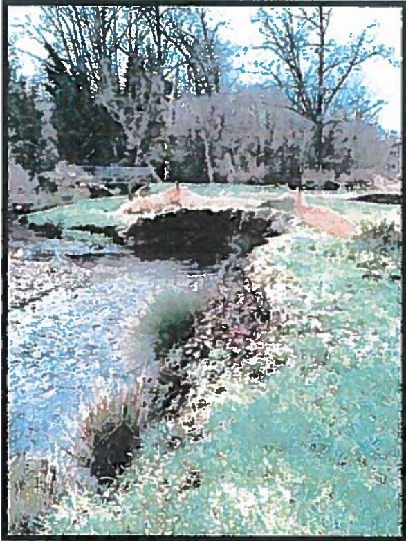
Bay City Al Griffin Memorial Park - Patterson Creek Streambank Erosion February 2022
